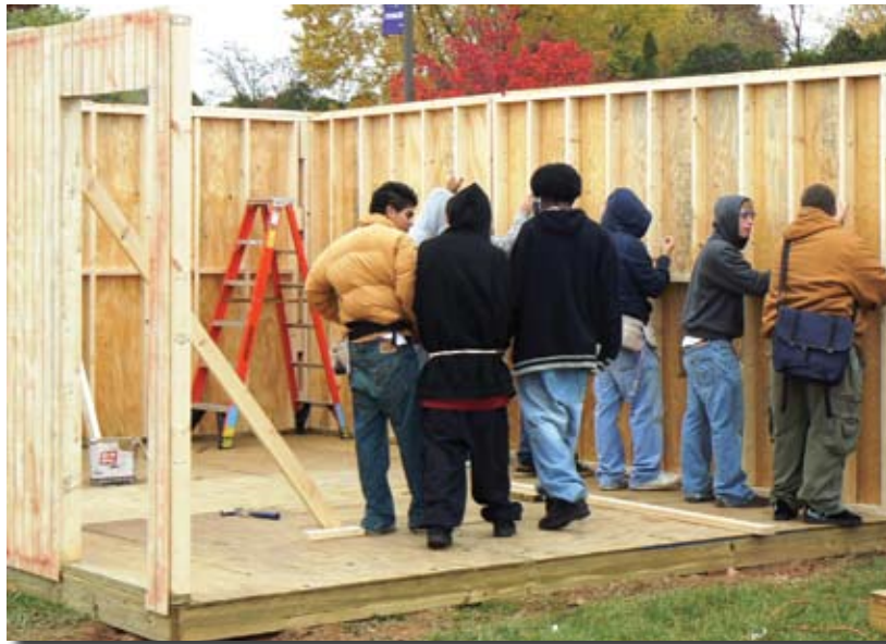
Construction Technologies students apply their technical skills in the construction of storage buildings for school and community customers.
